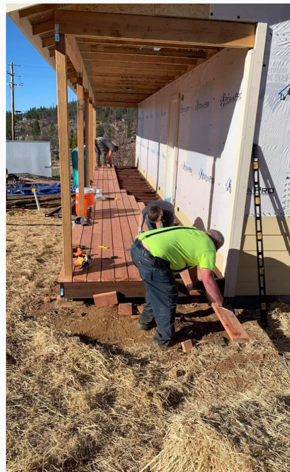
Wakarusa Missionary Church volunteers lay decking for the front deck on a rebuilt home
